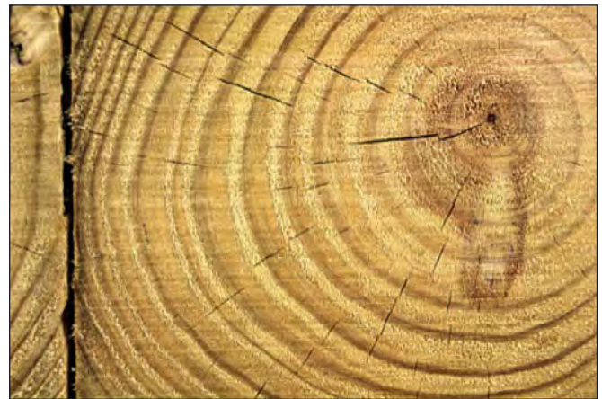
Figure 1. End checking of a pine timber.
