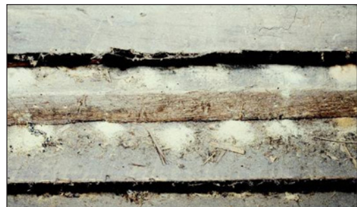
Figure 6. Powderpost beetle frass may accumulate in piles beneath exit holes.
