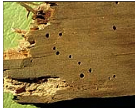
Figure 5. Wood damaged by powderpost beetles.
